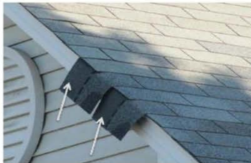
Asphalt shingles extending over eave.
